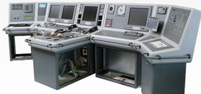
Platform electric comand center
